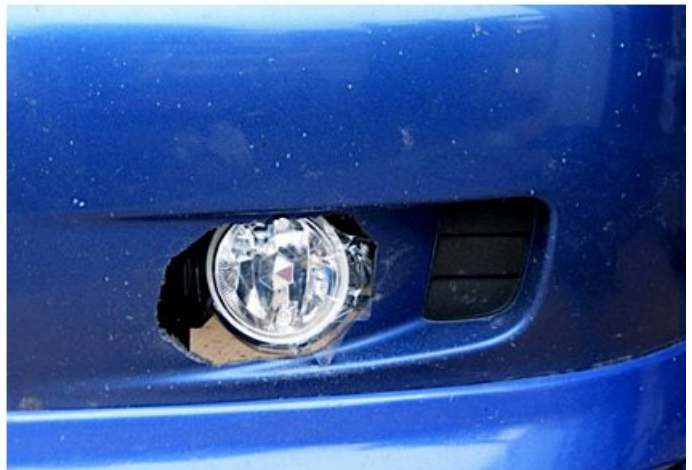
Here, the outside of the bumper cover in the previous photo is shown. It's always a good idea to use the fog light you'll be installing as a template. After drawing a line around it on the back side of the bumper cover, follow the lines as closely as possible when cutting.
